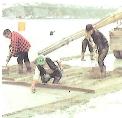
Exterior flooring with concrete admixed with PLANICRETE SP. Vieux Port, Quebec, Canada
